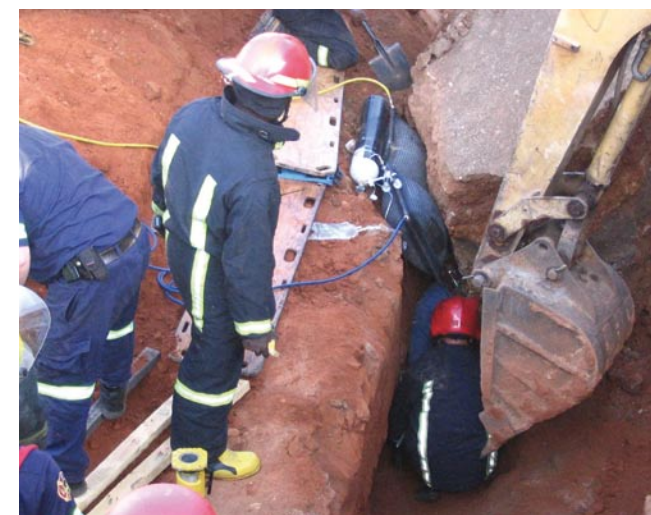
Trench collapse at Water World, Randburg, Johannesburg. During the extrications rain further destabilised the site, causing a second collapse (centre), which narrowly missed the rescuers
