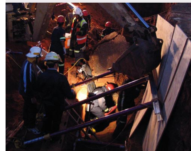
A round-the-clock operation followed the Water World trench collapse; two workers died and four were injured
